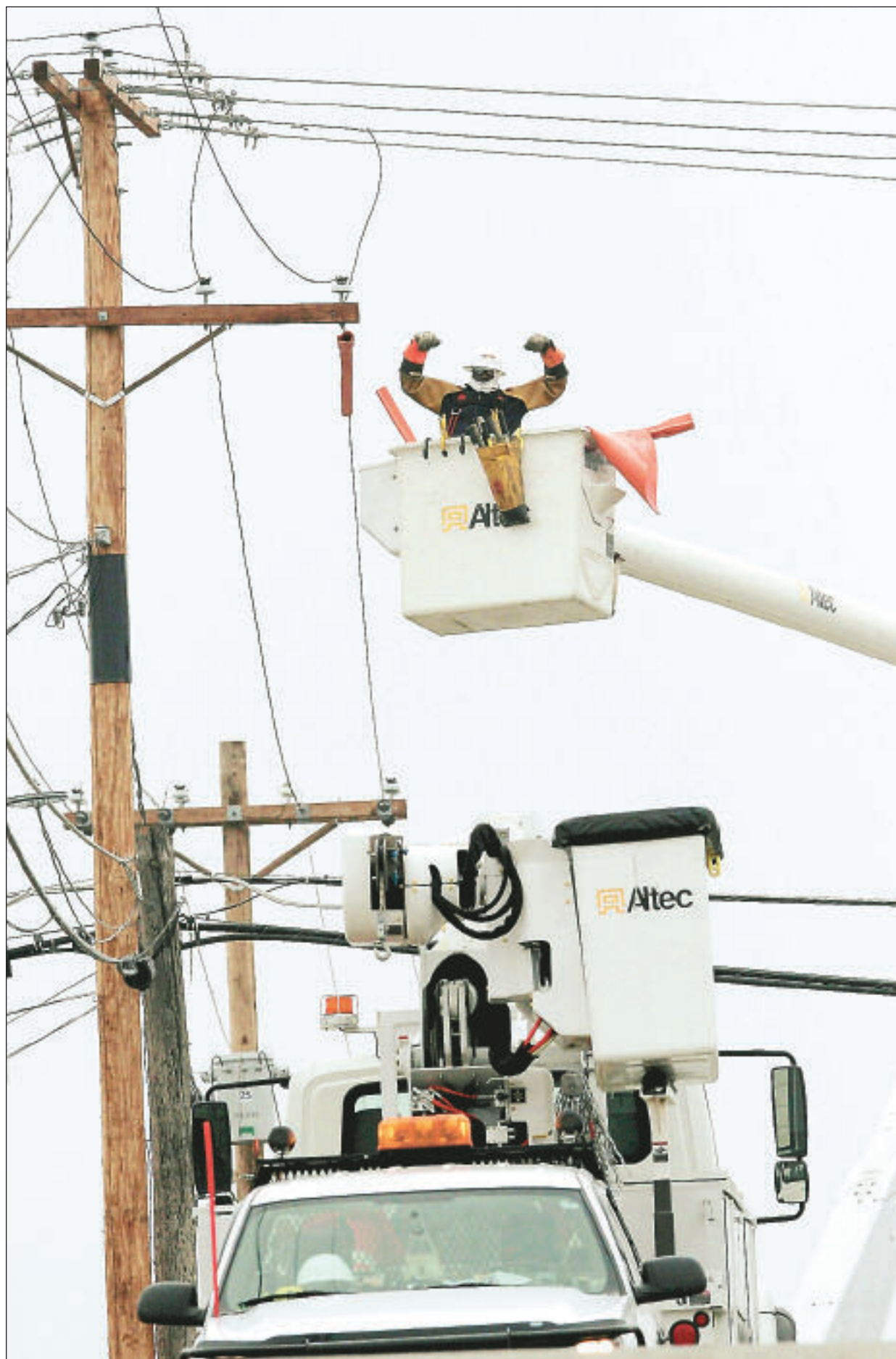
Chain Electric Co. lineman Leonard Robinson of Shreveport, La., signals success Friday after placing jumpers from a live power line to a dead line that serves an area in the 1900 block of 40th Street.
